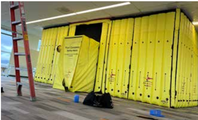
An example of a decon chamber.
