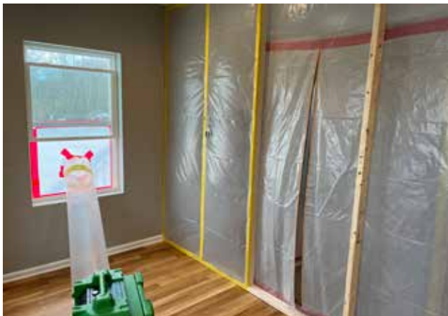
An example of venting contaminants out of a window.
